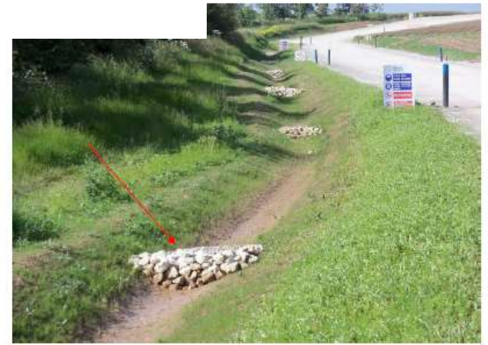
GP - SuDS with check dams installed and maintained and good vegetation from grass seed as per Ecology Plan
